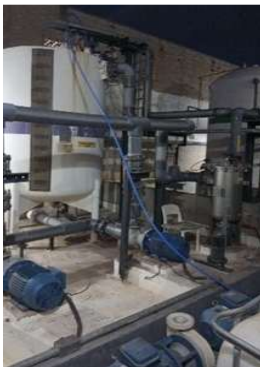
Figura 138: Tanque e Bombas de CIP (Clean In Place)
